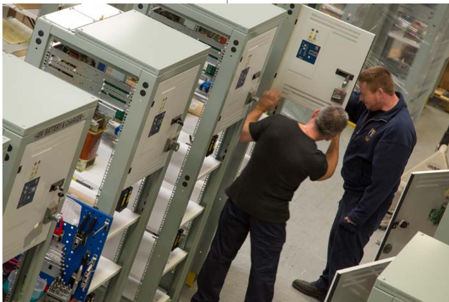
PB Design has produced tens of thousands of battery charging systems since its inception
